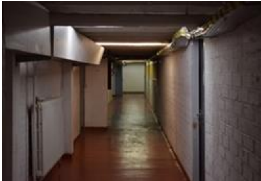
Figure 13. Photograph of the corridor in the basement of the late-1950s building, after expansion in 1959. Picture by author (2021).
